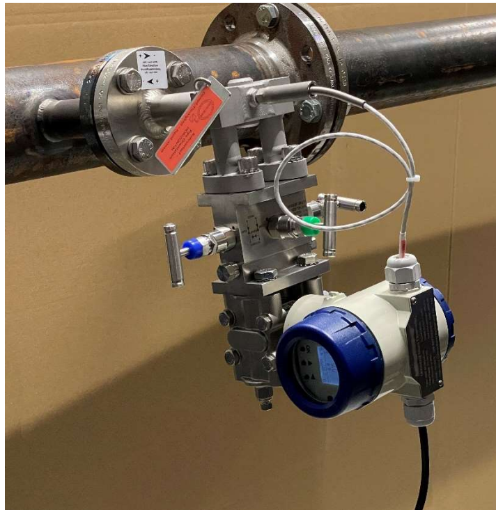
deltaflow DF25 for with integrated PT100, condensate trap, three-way block and SYS-MMF in a horizontal DN100 steam line
